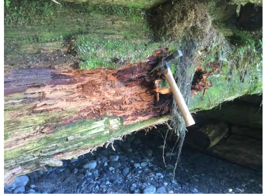
Stringer 7 Midspan Sap Rot & Bug Infestation
