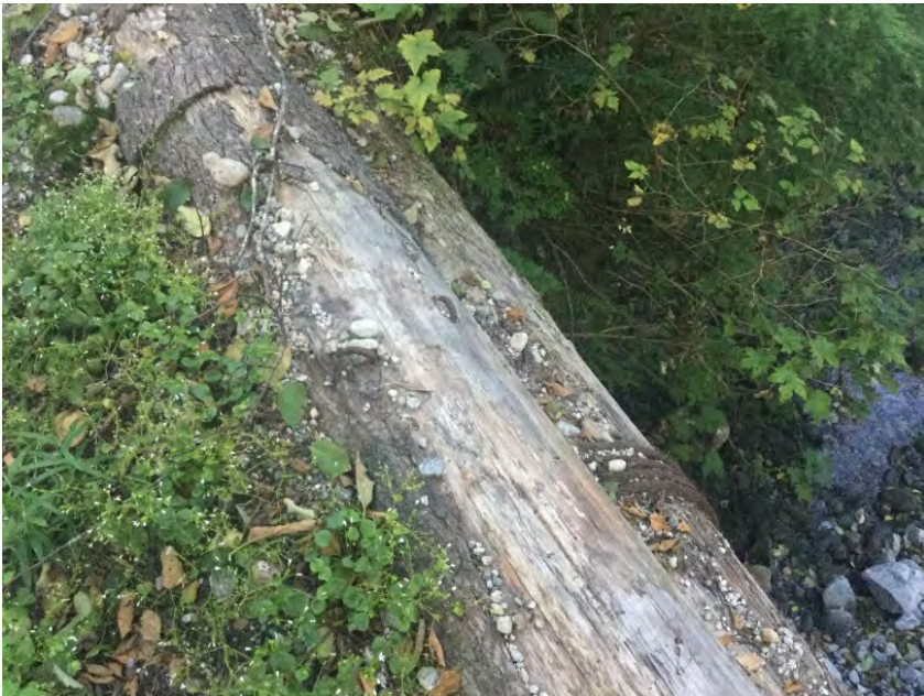
Missing Log Curb Lashing Left Abutment Downstream Corner.
