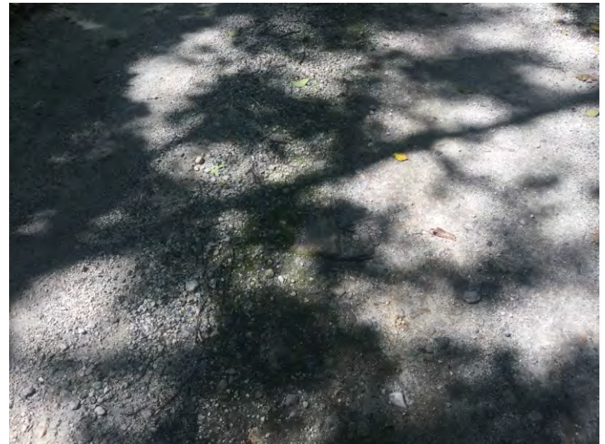
Left Abutment Exposed Stinger in Centre of Road
